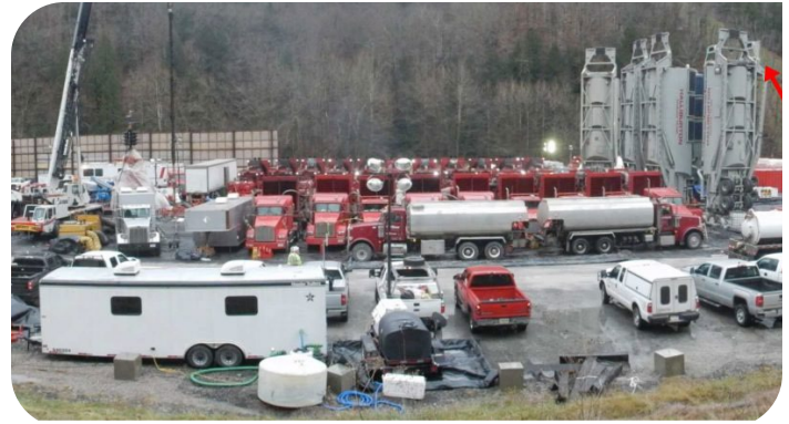
Fracking Well Site in Wetzel County, West Virginia Source: Ohio Valley Environmental Coalition
